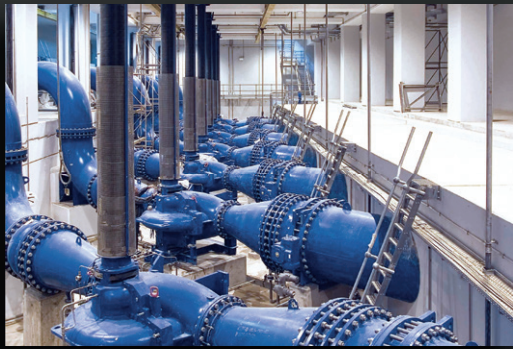
Pumps and compressors
